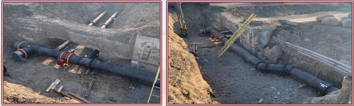
18" diameter HDPE Central Loop
