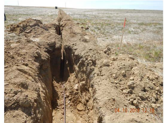
Plugged and abandoned well encountered and exposed during excavation work (view to South)
